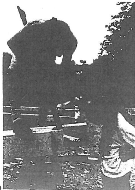
10 A sense of the heaviness of the work when manipulating timbers precisely. In the background is the indented surface of a timber finished with an adze.
